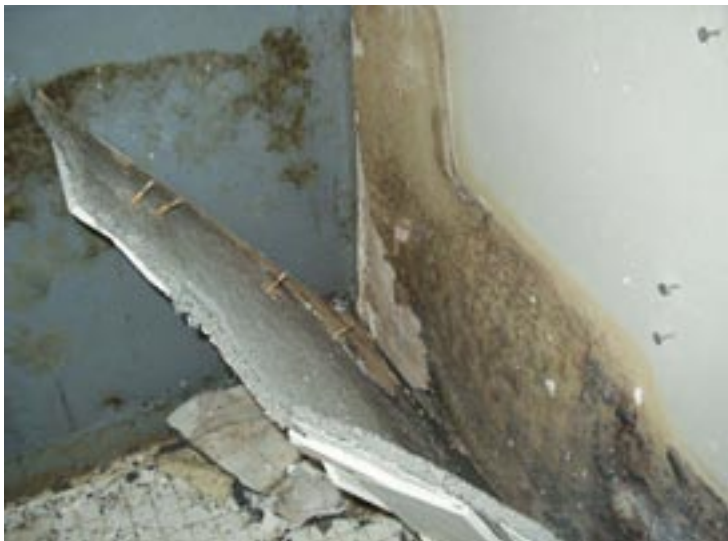
Figure 2. No waterproofing was used in this shower.
