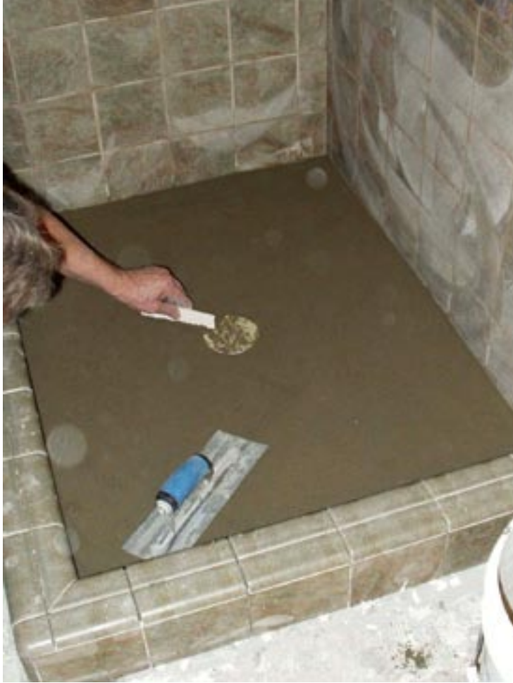
Figure 1. The shower pan is below the mortar.
